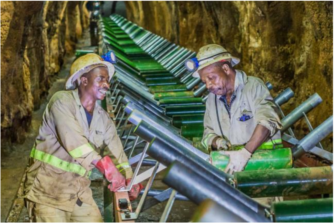
Figures 6 and 7: Installation of conveyor belt rollers in Shaft 5 ore load-out system.
