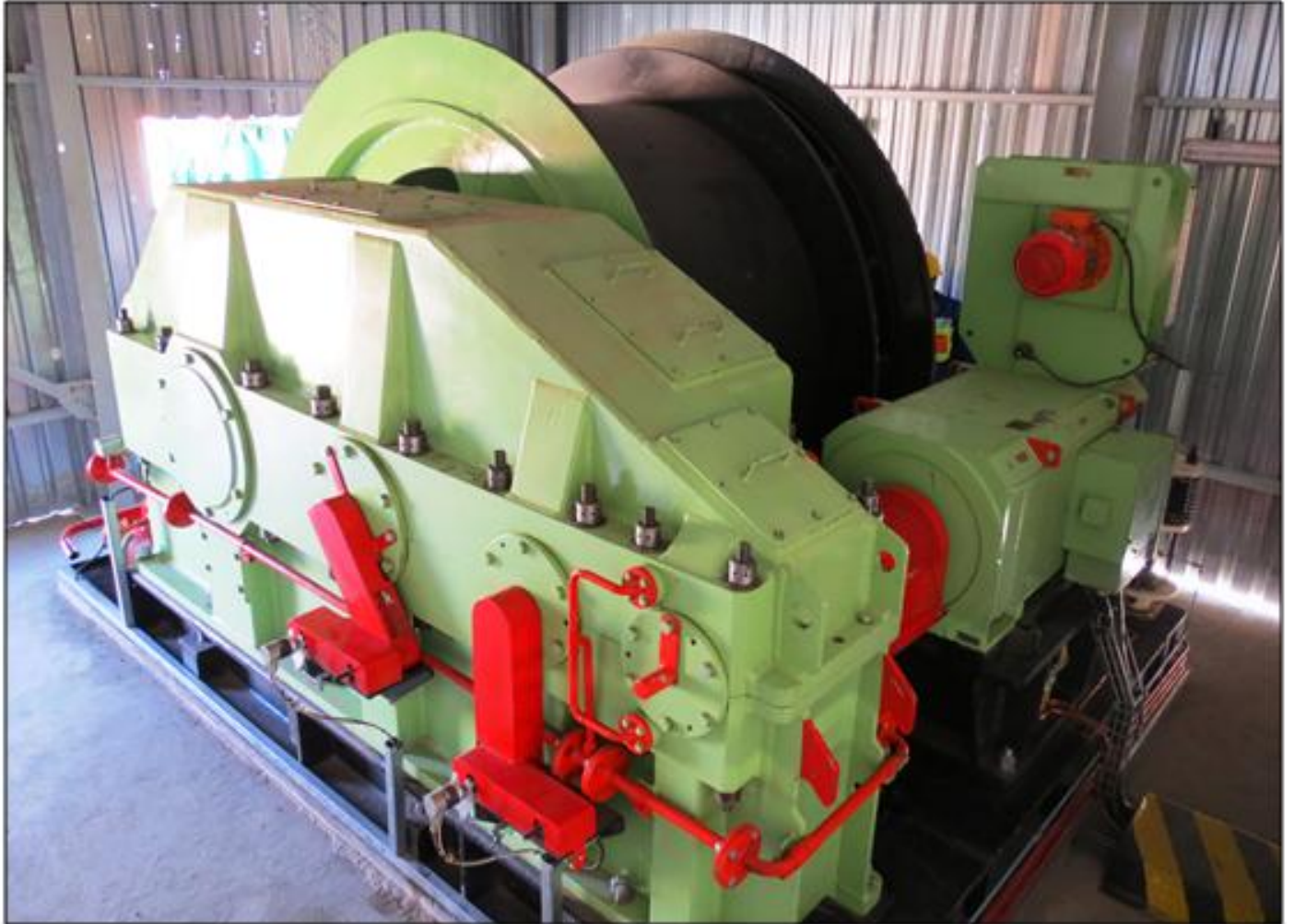
Figure 4: Pre-sink winder installed.
