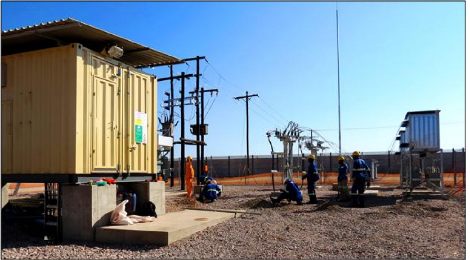
Figure 5: 5MVA sub-station and lines to deliver Eskom power.
