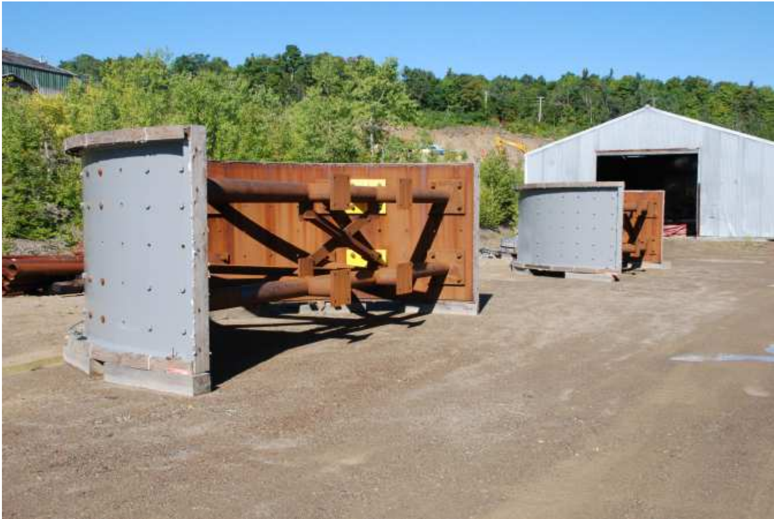
Figure 2: New 3,000-tpd SAG mill and components are onsite for installation in the Caribou Mill
