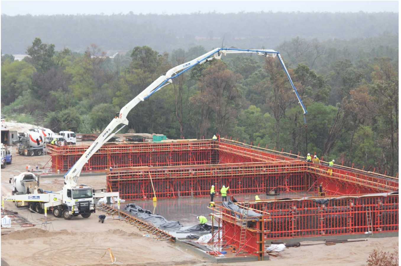
Pouring concrete for new finished product stockpile as part of the Stage 2 Expansion at the Greenbushes Lithium Operations.
