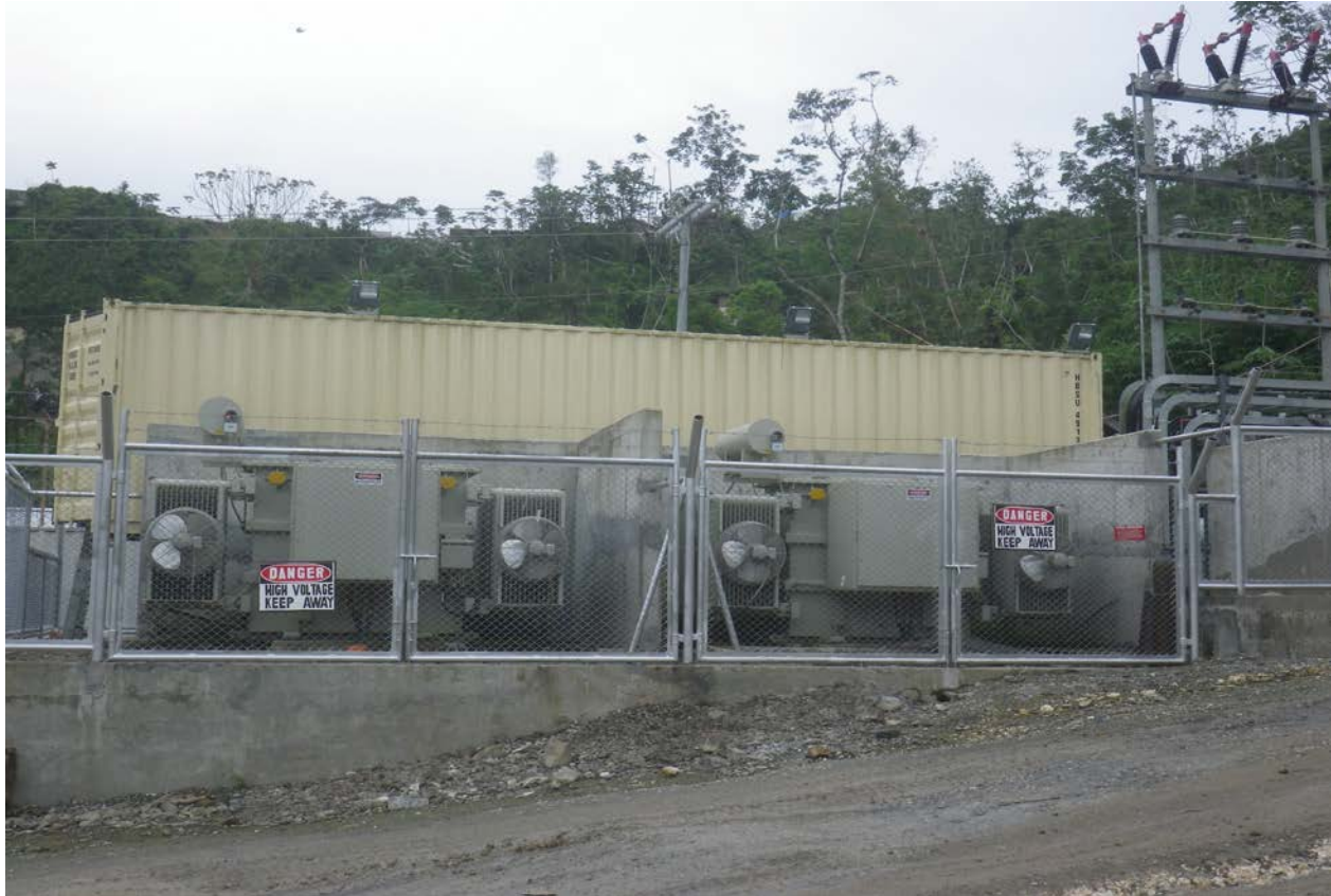
Photo 5. Mine transformer station.
