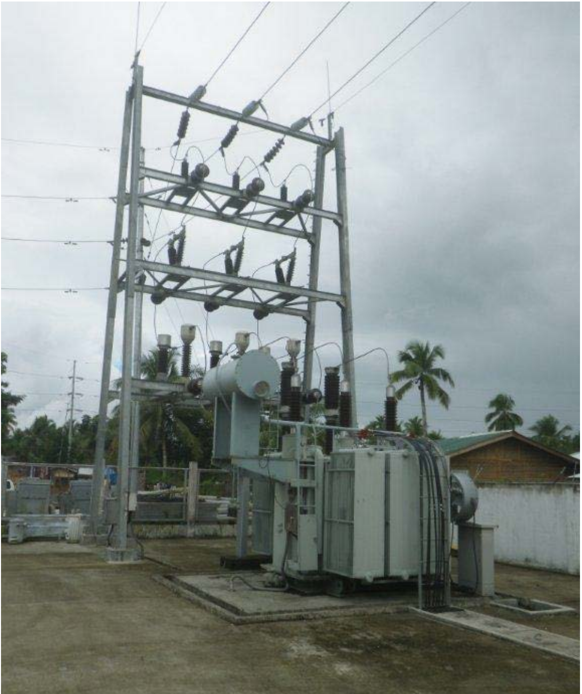
Photo 6. Mill transformer station
