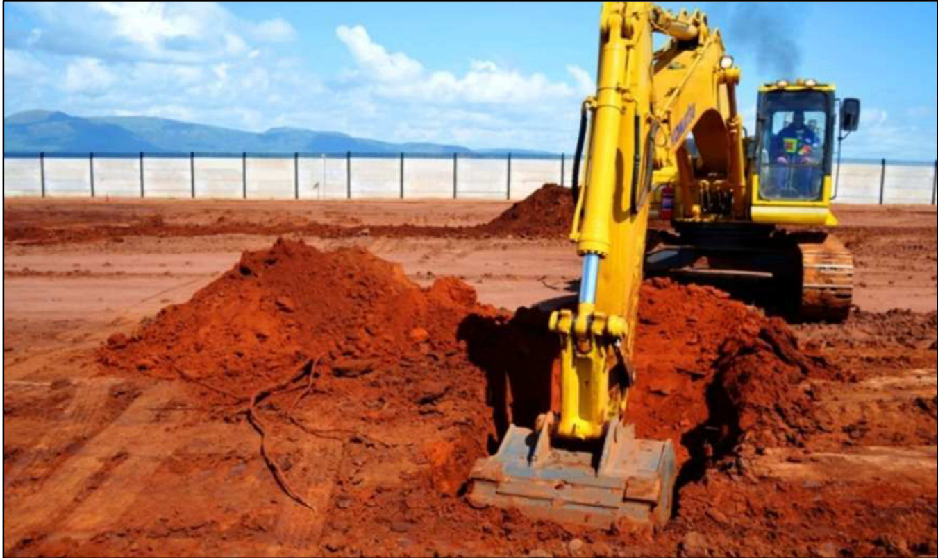
Figure 2: Box-cut excavation in preparation for sinking of bulk-sample shaft at Platreef Project.
