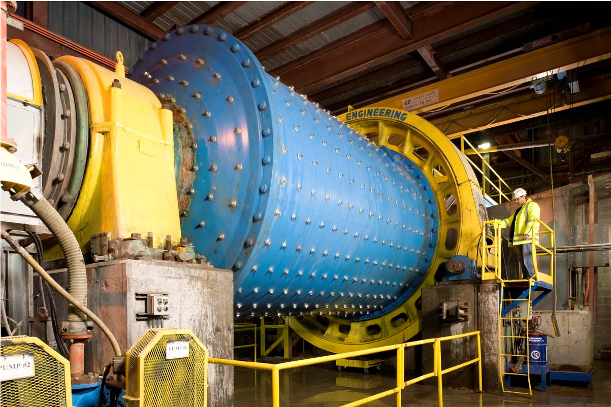
Below is a photo of the Bell Creek Mill's primary ball mill in operation.
