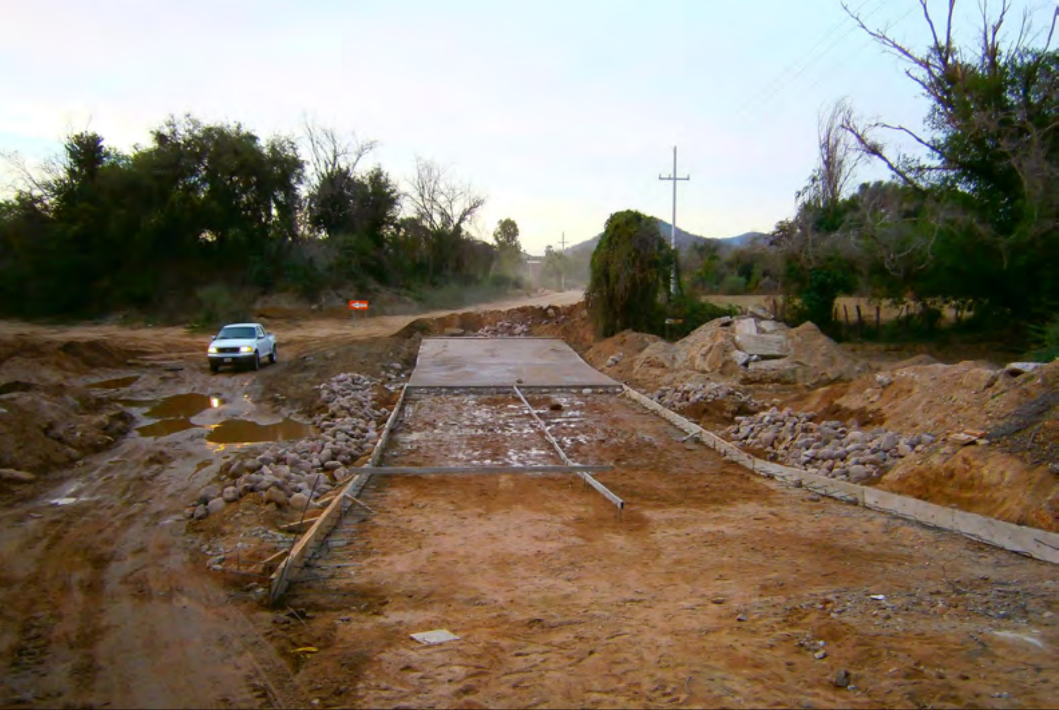
Bridge under construction. Haul road will connect the Palmarito and El Gallo deposits.
