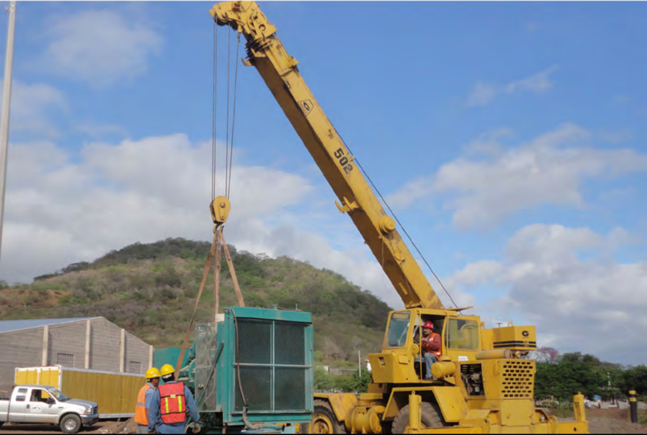
Replacing generators that will be used to power the crushing plant.
