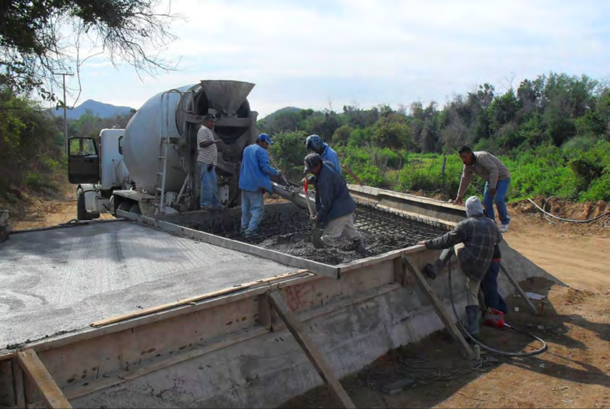
Bridge construction along the haul road between the El Gallo and Palmarito deposits.
