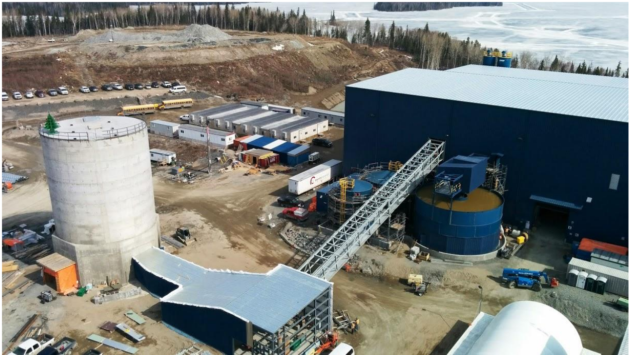
View of the completed crushed ore bin, construction of the conveyor system, and mill thickener outside the mill building.
