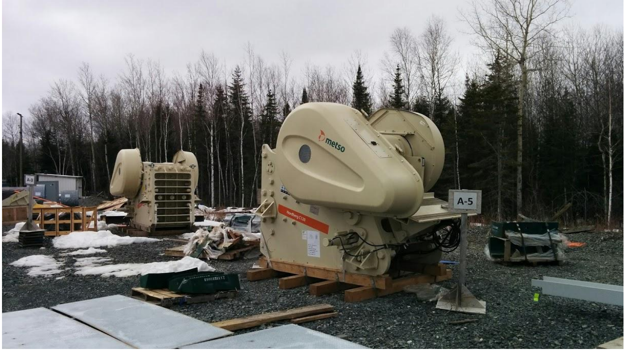
Underground crusher on site in preparation for installation above the 305-metre level
