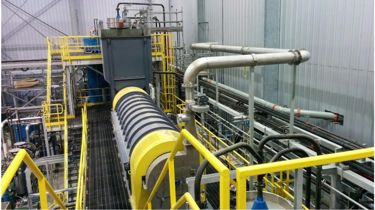
Carbon elution plant commissioning
