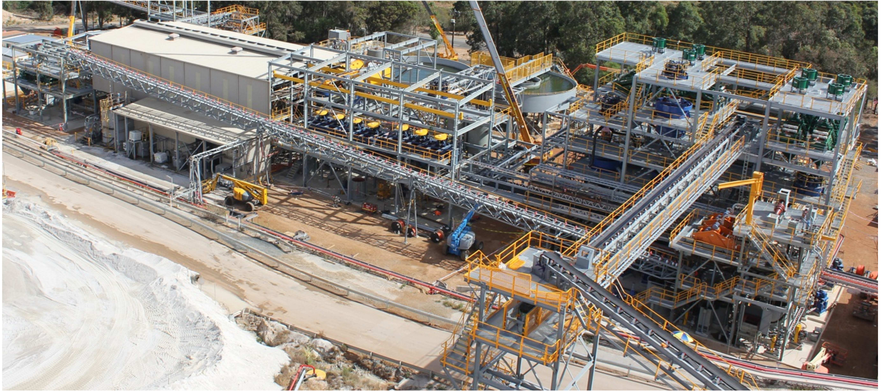
Work on the new chemical-grade plant as part of the Stage 2 Expansion at the Greenbushes Lithium Operations.
