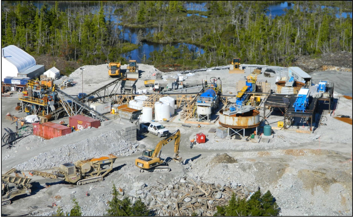
Figure 1 – Yellow Giant Process Plant – July 1 st 2014
