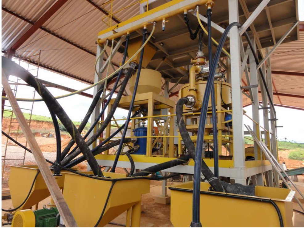
Gekko Gravity Concentrating Plant at Sao Chico
