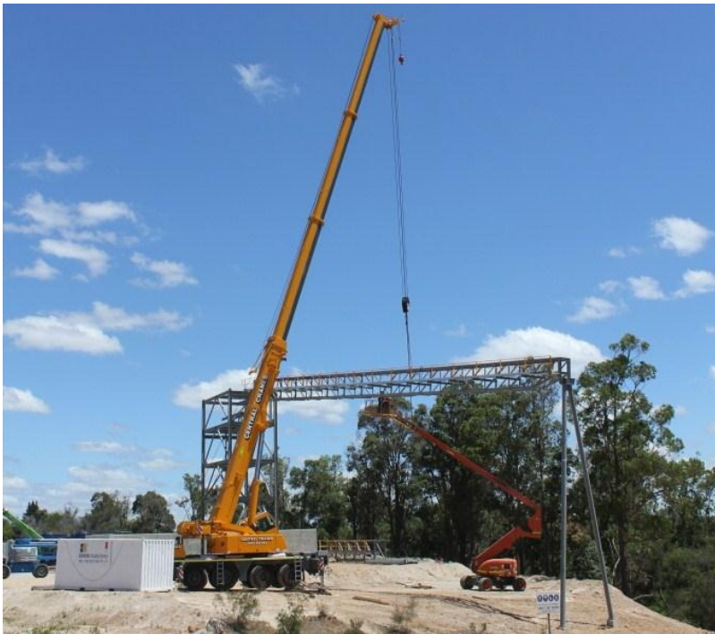
Conveyor belt to finished product stockpile being constructed as part of the Stage 2 Expansion at the Greenbushes Lithium Operations
