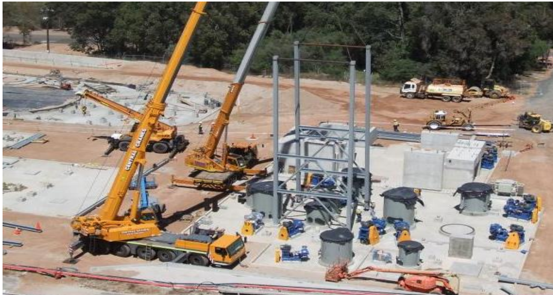
Commencement of steel-work as part of the Stage 2 Expansion at the Greenbushes Lithium Operations.
