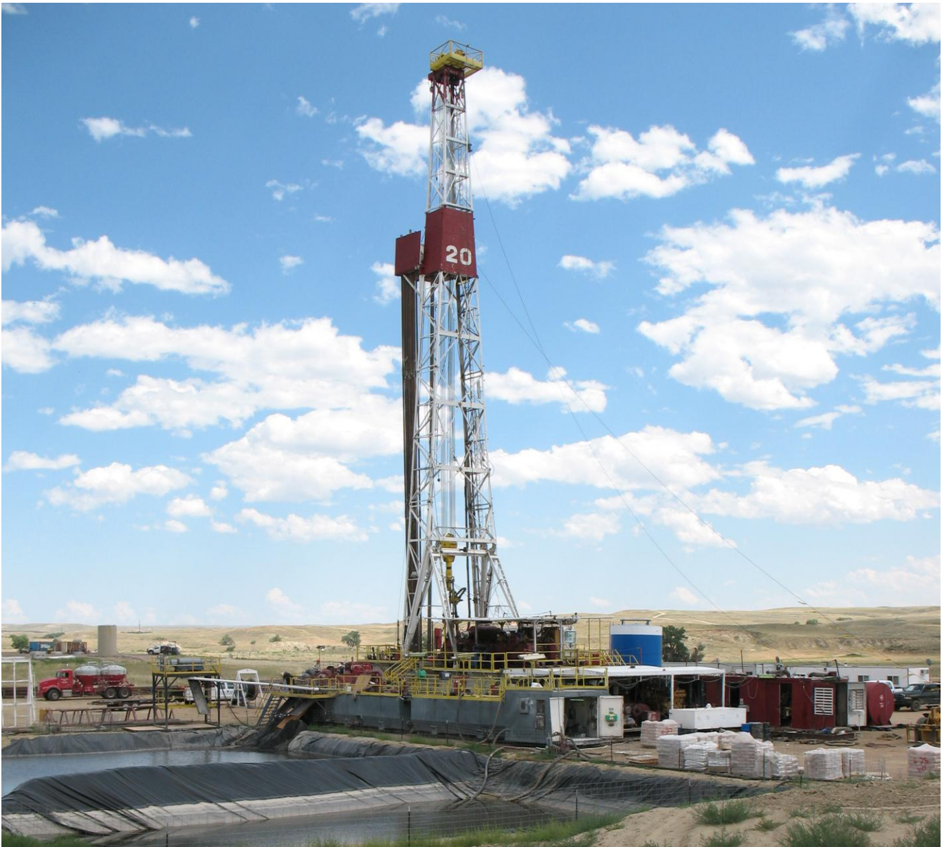
Drilling rig at the first deep disposal well site of the Nichols Ranch ISR Uranium Project.
