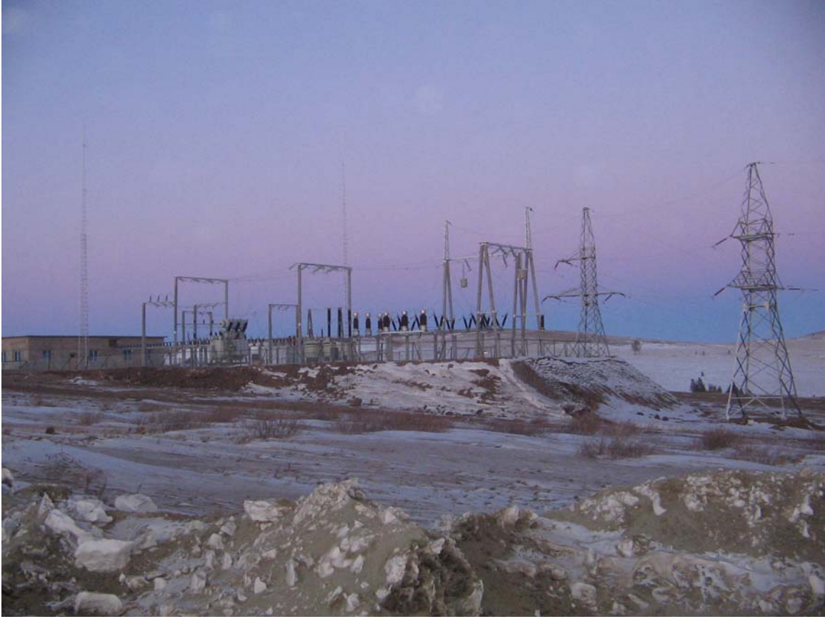
Figure 1 - Electrical substation at Gurvanbulag, Mongolia
