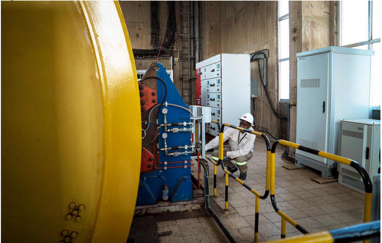
Figure 10: Shaft 5 hoisting winder.
