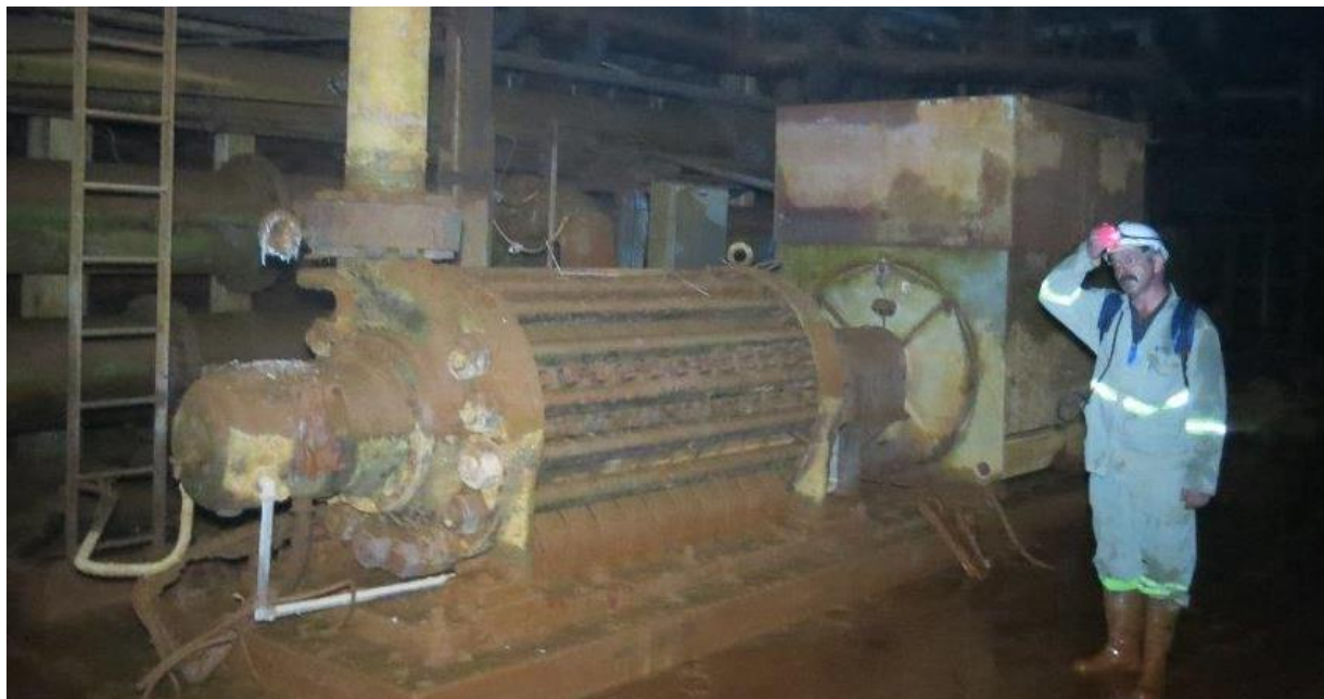
Figure 8: One of five existing high-capacity Sulzer pumps in the main pumping station that will be refurbished.
