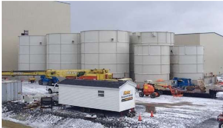
CIL & Detox Tank Installations
