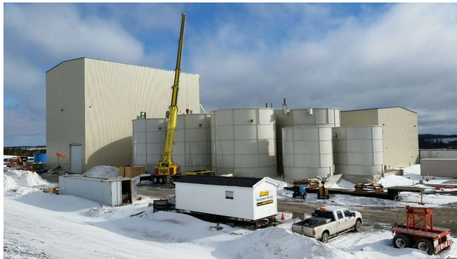
CIL tanks and cyanide destruction tanks complete
