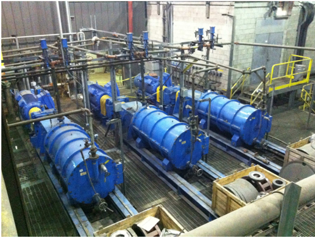
Figure 2: Three M1000 IsaMills installed at Trevali's Caribou mill
