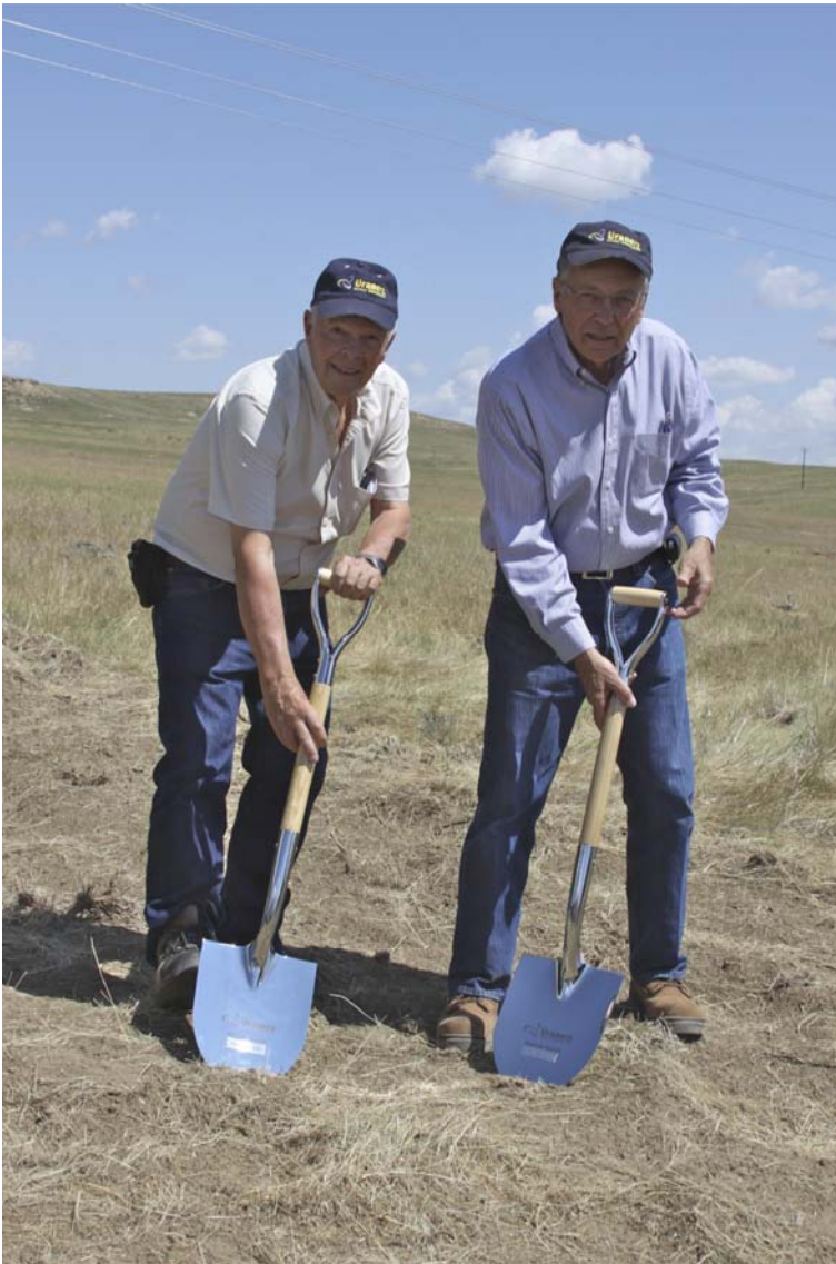
In photo: President & CEO, Glenn Catchpole (Right) Executive VP, COO, George Hartman (Left) insert ceremonial first shovels into the ground.
